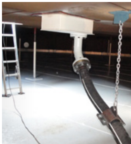
CTS tank drain hose at centre sump.
