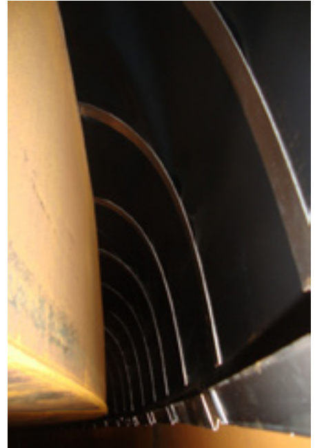
STT Belgium CTS30 primary seal on steel floating roof.
