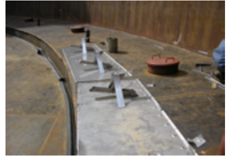
CTS1 scissor type shoe plate seal with energised hangers, ready to be fitted.
